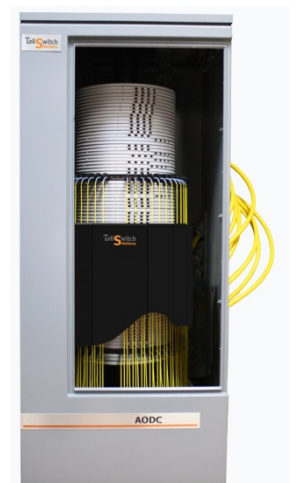
AODF-MN Frame Front View
